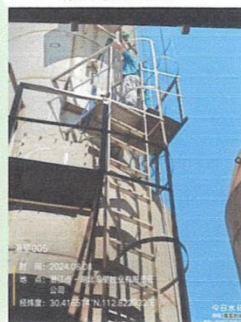
车间废气排气筒DA005
